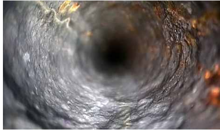
Real life problem 2 Corrosion of Piping
